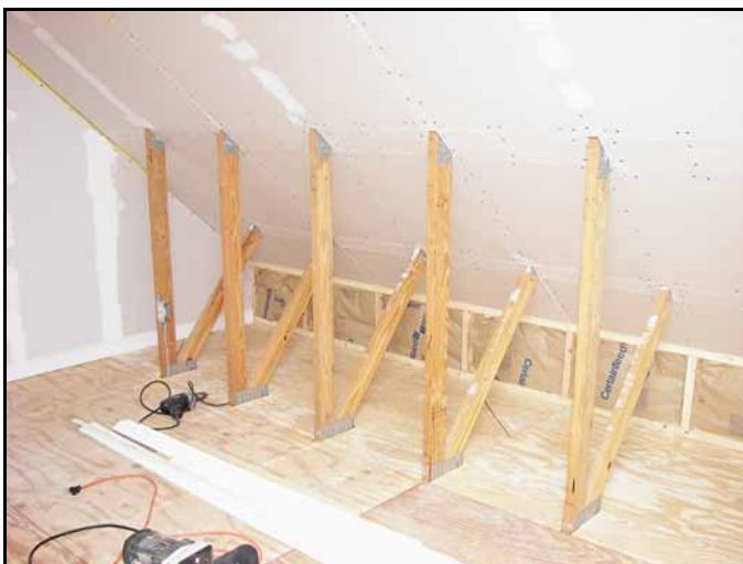
It took some time to carefully measure and cut each section of wallboard and then form fit each piece into place to get a tight fit. Adding wall mud to all the seams was a real challenge.
