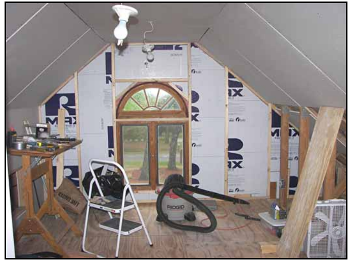
The existing window wall was insulated with several layers of 3/4 inch foam insulation. Once the insulation phase was complete I started adding the wallboard to the ceiling and then the walls.
