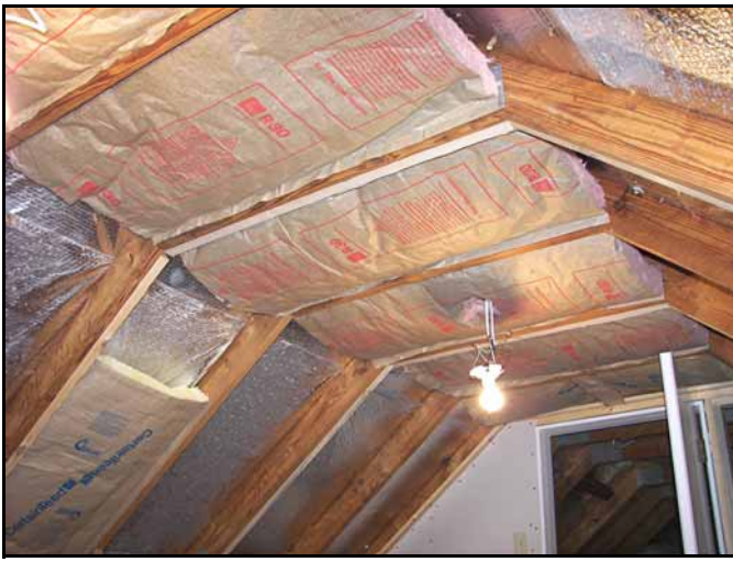
Once all the framing was completed it was time to insulate the ceiling and the walls. I used R-30 for the ceiling and R-11 for the walls.
