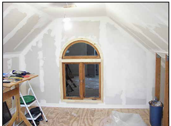
I added fiberglass mesh tape to the seams and corners and then gave them 2 coats of mud. I added the trim work and then I diluted the mud a bit so that it would flow better and I applied it to the entire surface of the ceiling and the walls.
