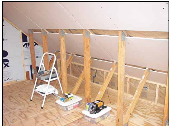
I added small sections of 3/4 inch pine strips to the left and right sides of each opening between the trusses so that the small sections of wallboard would be securely screwed into place.
