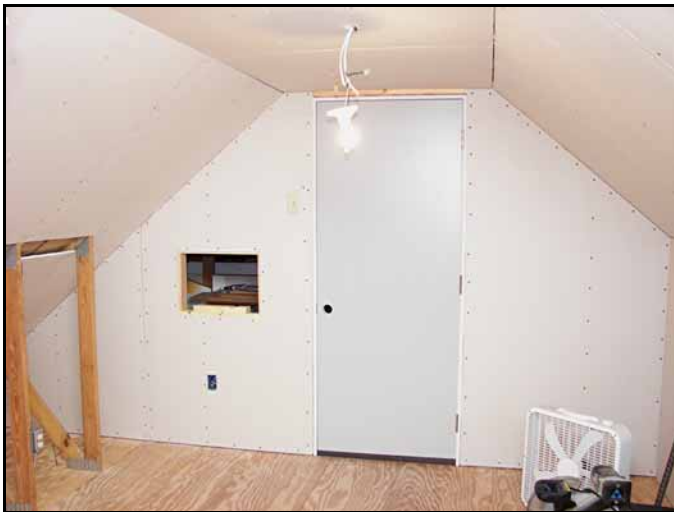
My sons Tom and Greg helped me position the wallboard and I used screws to attach the sections to the framing. I carefully measured and cut so that the joints would be tight. Unfortunately the ceiling joints had some gaps!
